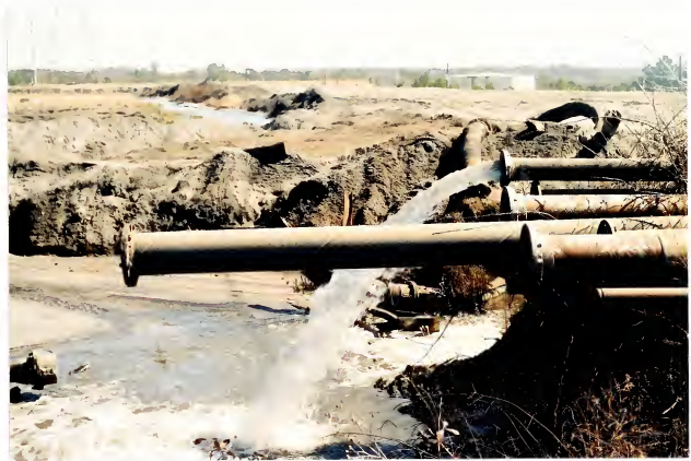
Figure 17. Permitted Discharge from Plant McDonough. The discharge pipes shown above are the outlets of the discharge from the plants two boilers. Two of the pipes carry fly ash and two carry bottom ash. Others carry storm runoff from the coal stockpiles. This co-mingling of wastes makes it difficult to utilize the CCBs for beneficial purposes as it would require sieving to separate the fly ash from other wastes. Not pictured here is the sulfite (from the sulfur injection system), found in a pile near the center of the pond, it is another co-mingled waste.
